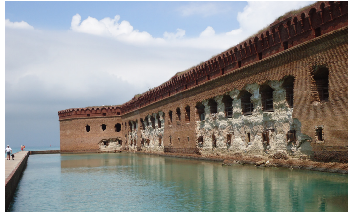
At Dry Tortugas National Park, repair planning at Fort Jefferson must take into account projected sea level rise and increased storm intensity.
